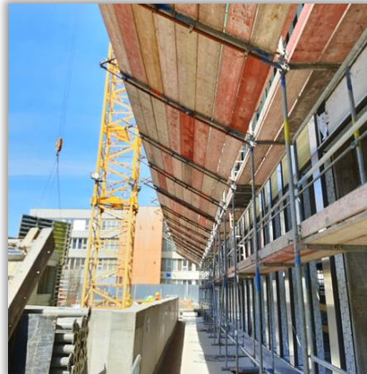
Protective roof along the communication road Face2Face
